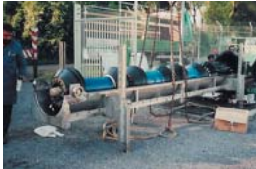
26-inch pig trap with intelligence pig for crack detection measurement
