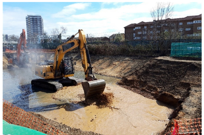
Figure 8: Photo showing the excavator adding the oxygenating compound. The machine used for subsequent mixing is seen in the background.
