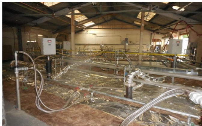
Figure 2: Heating and recovery well array.
