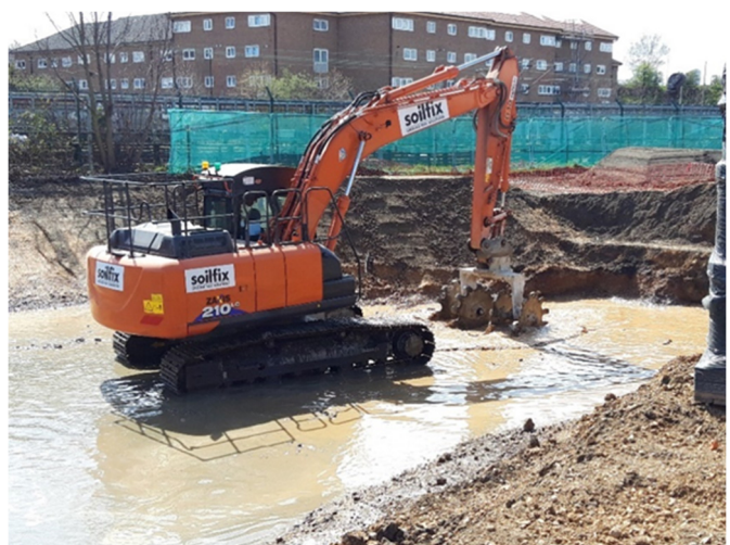
Figure 9: Photo showing mixing the reagent into the top layer of material using a specialist attachment on the arm of the excavator.
