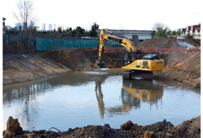
Figure 7: Photo showing that the depth of the dig was just beneath the groundwater level to reduce over-excavation.
