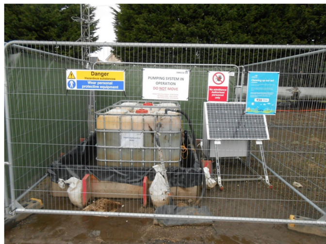
Figure 4: Remediation system at BHS17-04A.
