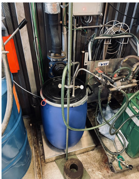
Figure 5-6 Fuel scale and test fuel rig.
