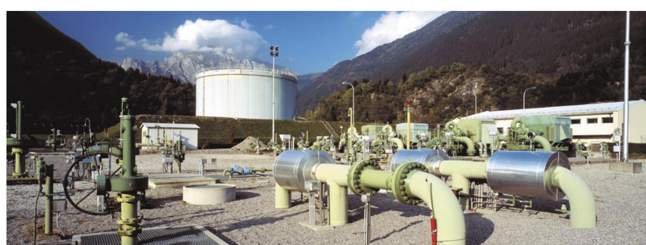
Pump station, Paluzza (Italy)
