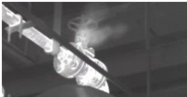
Figure 4 An image of a leak otherwise not visible to the naked eye
